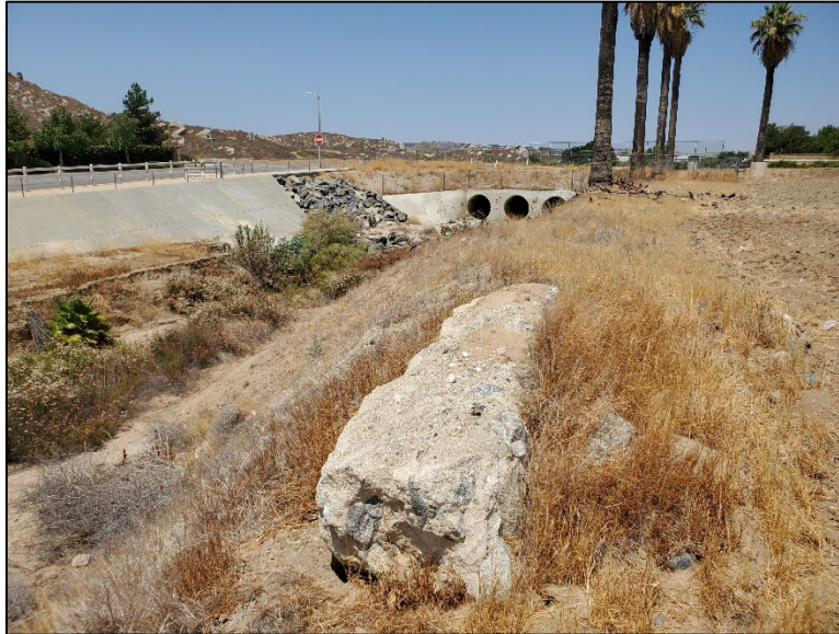
Figure 16. Overview of concrete drain system in northwest corner of Project, view northwest
